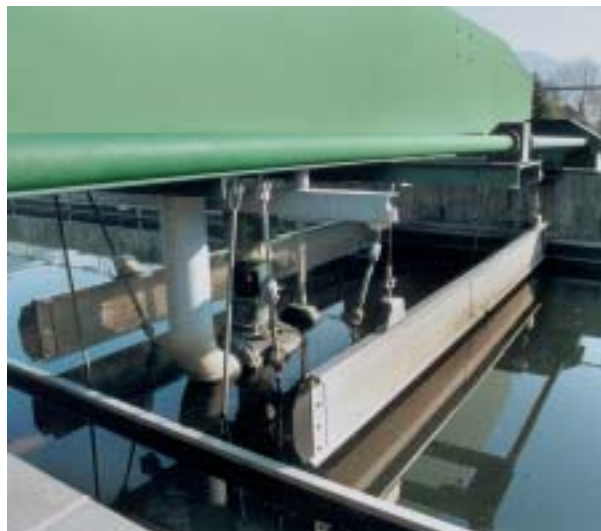
Returned sludge pump installed on a rotating scraper bridge.
